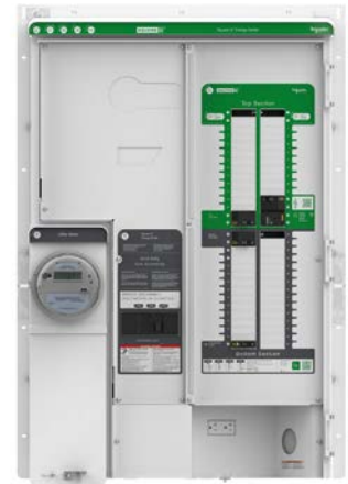
Energy Center with Cover Removed
