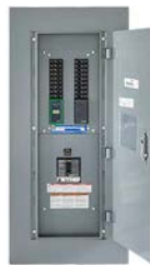
NQ MB Panelboard with SurgeLoc SPD installed
