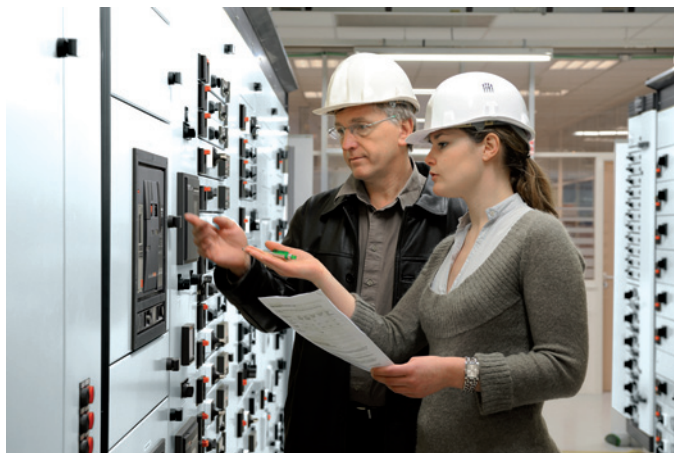
Motor Control Centre (MCC).
