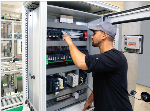
General machine control
