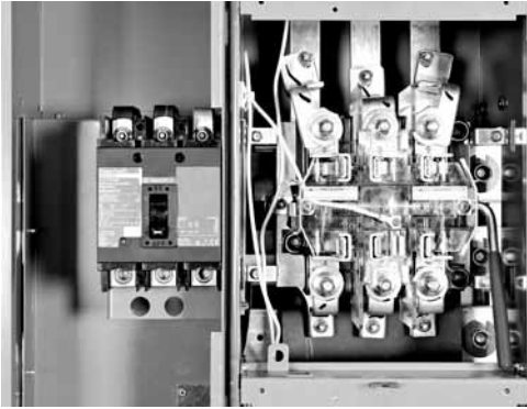
Q-Frame Circuit Breaker Installed
