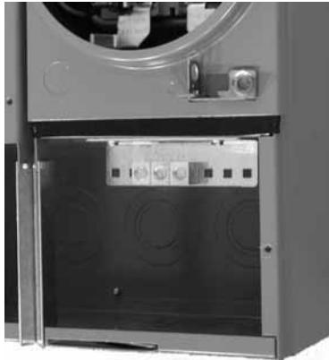
Branch Unit Load Equipment Grounding Terminals
