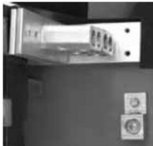
Grounding Lug and Isolated Main Neutral Bus as Installed at Factory on Main Devices
