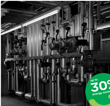
ATV12 drive controlling a pumping station
