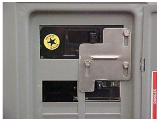
Generator Interlock Kit (In use)
