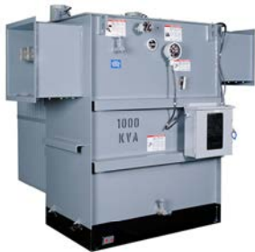
Liquid Filled Substation
