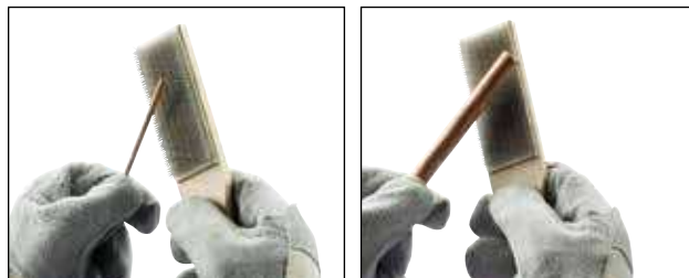
Fig. 5 Next, use a wire brush to further prepare the surface of the conductors and ground rod (Cadweld T-313 or T-314 brush). Scrape the outer surface to remove dirt and oxidation. You will notice a slight color change.
