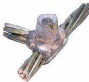
Reject. Extreme amounts of slag on surface are caused by welding material leaking past disk or complete lack of disk. Inspect the condition of mold disk seat and check disk positioning prior to making the next connection.
