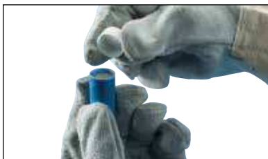
Fig. 10 Next, take the tube of welding material included in the Cadweld One Shot package and remove the lid over the crucible.
