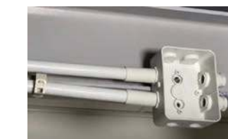
Conduits & electric box from beam
