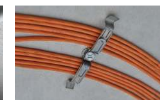
Cables from concrete ceiling / wall
