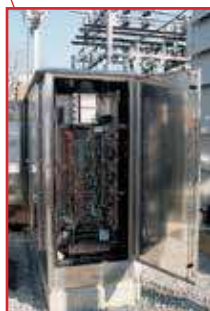
Power and Control Surge Protection for SCADA and Power Connections
