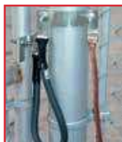
Fence and Gate Jumper Assemblies
