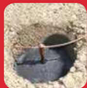
2. Ground enhancement material, GEM or Quickfill
