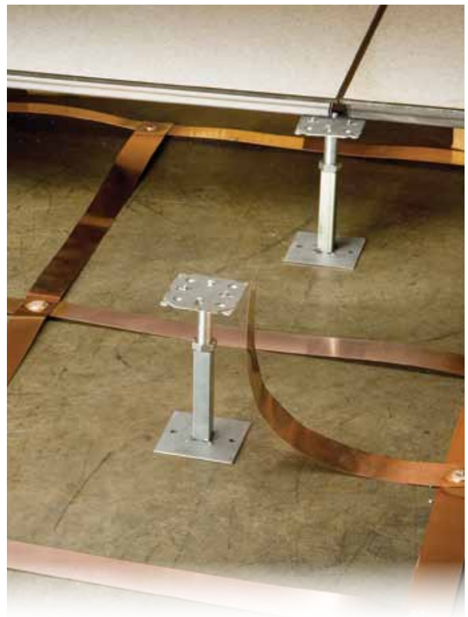
Pre-fabricated Signal Reference Grid installed under computer room floor.
