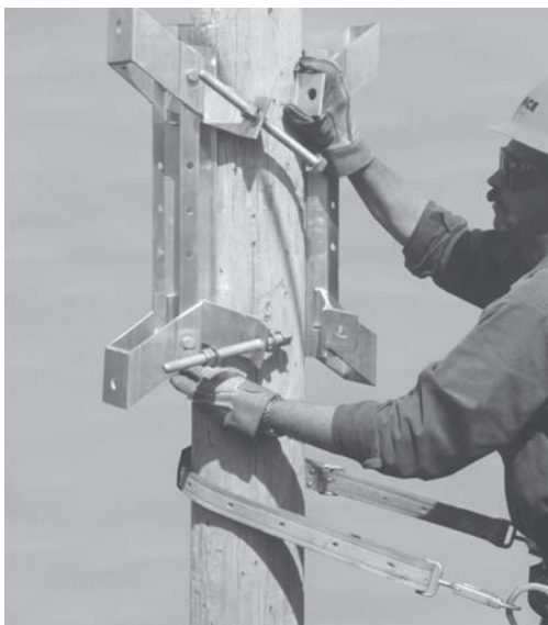
3. Use a lag screw installed into the pole to locate where you want the cluster mount positioned. The lag screw is used for positioning only and not to bear the load.
