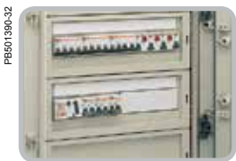
Detail from the circuit-marking system.
