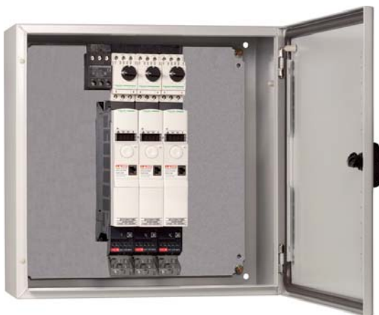
Example of GV2/Altivar 32 direct mounting in an enclosure: GV2 P self-protected disconnect + GV2GH7 line spacer + ATV 32HU15N4 drives
