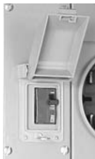
Circuit Breaker Cover, Open
