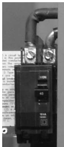
QO2100 Plug-On Circuit Breaker Installed
