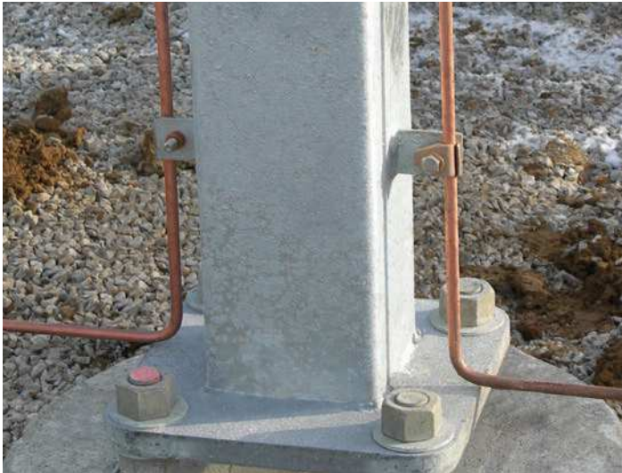
Substation earthing riser
