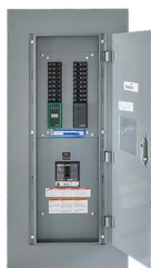
NQ MB Panelboard with SurgeLoc SPD installed
