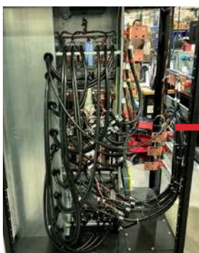
Cabinet with cables
