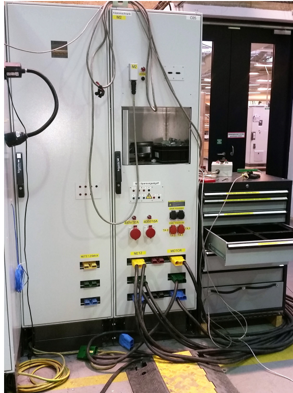
Figure 3 Main Disconnect and Terminations
