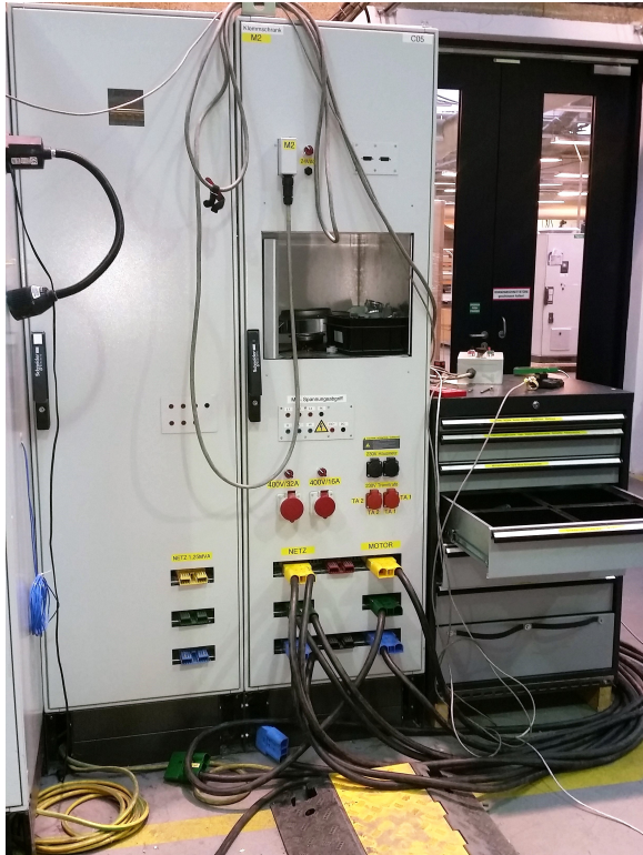
Figure 3 Main Disconnect and Terminations
