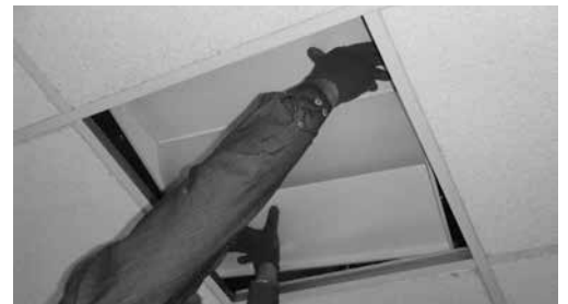
Step 6 Adjust fixture to sit properly in grid. Ensure fixture is installed based on the local codes.
