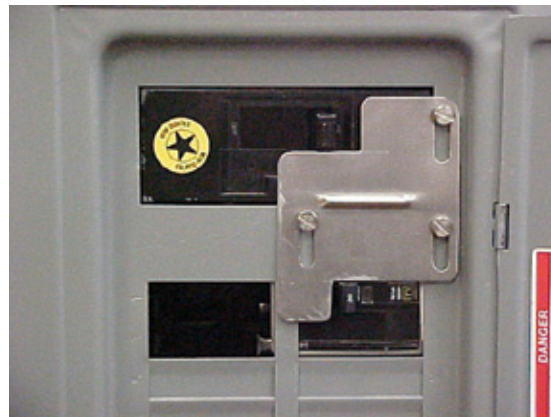
Generator Interlock Kit (In use)
