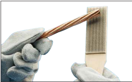
Fig. 12 – Next, use a wire brush to further prepare the surface of the conductors (nVent ERICO T-313 or T-314 brush). Scrape the outer surface to remove dirt and oxidation. You will notice a slight color change.
