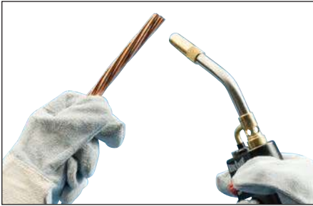
Fig. 11 – The conductors should be clean and dry before the connection is made. Use a propane torch to dry wire conductors and remove remaining cleaning residue, solvent, or water before making the Cadweld connection.
