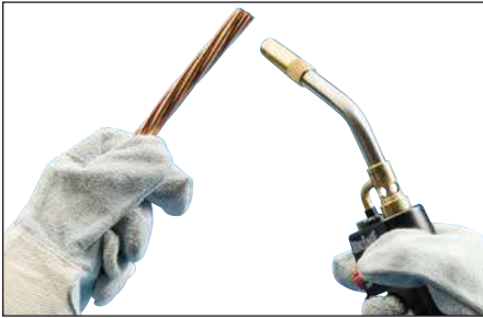
Fig. 11 – The conductors should be clean and dry before the connection is made. Use a propane torch to dry wire conductors and remove remaining cleaning residue, solvent, or water before making the Cadweld connection.
