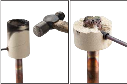
Fig. 15 – Break the ceramic Cadweld One Shot mold off of the connection. Avoid contact with hot materials. See the “nVent ERICO Cadweld Quality Standards” section to see whether a quality connection has been made.
