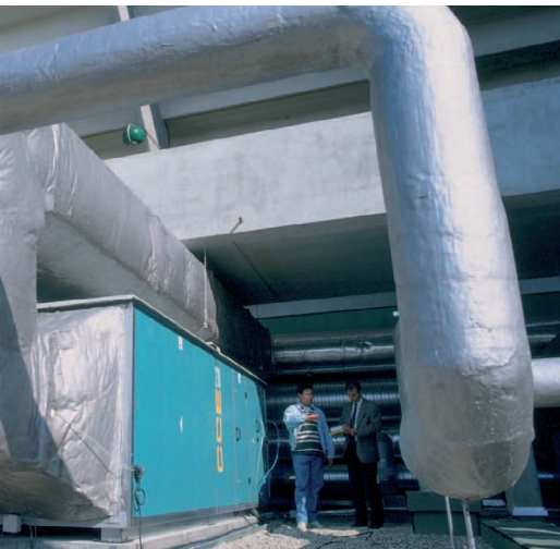
Circulating pumps for building management
