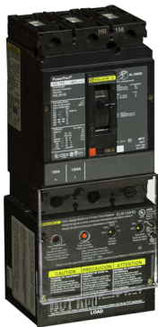
I-Line J-Frame with ELM Installed
