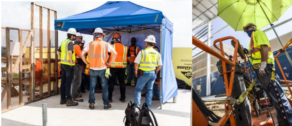
PORTABLE WORK SHELTERS
