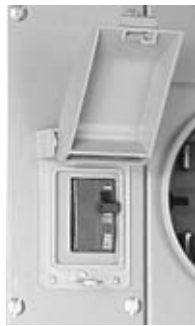
Circuit Breaker Cover, Open
