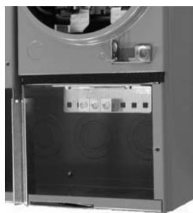
Equipment Grounding Lugs
