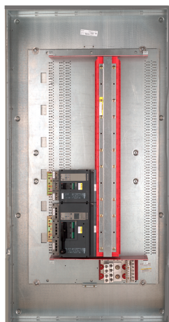
Type HCR-U— 1200 A Main Circuit Breaker
