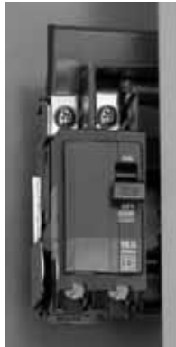
QO2100 Tenant Circuit Breaker Installed
