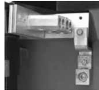
Service Grounding Lug, Bonding Strap, and Bonded Main Neutral Bus as installed on Main Devices at Job Site as Required for use as Service Equipment
