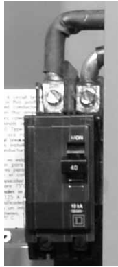
QO2100 Tenant Circuit Breaker Installed
